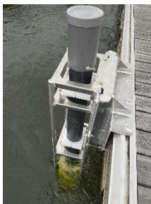
Figure 1 : Station SYVEL de Pierre Percée
